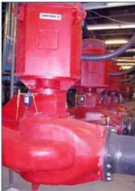
Enwave District Cooling Facility, Toronto, Canada.
