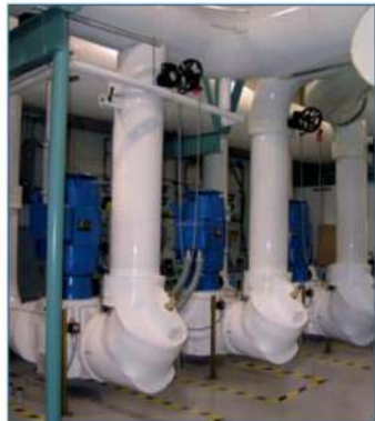
District Cooling Project, Phoenix, U.S.A.
